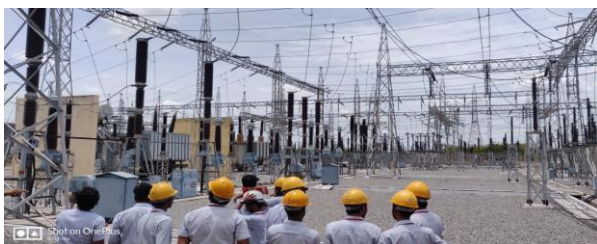
220KV/132KV/33KV Substation, Chillakallu
